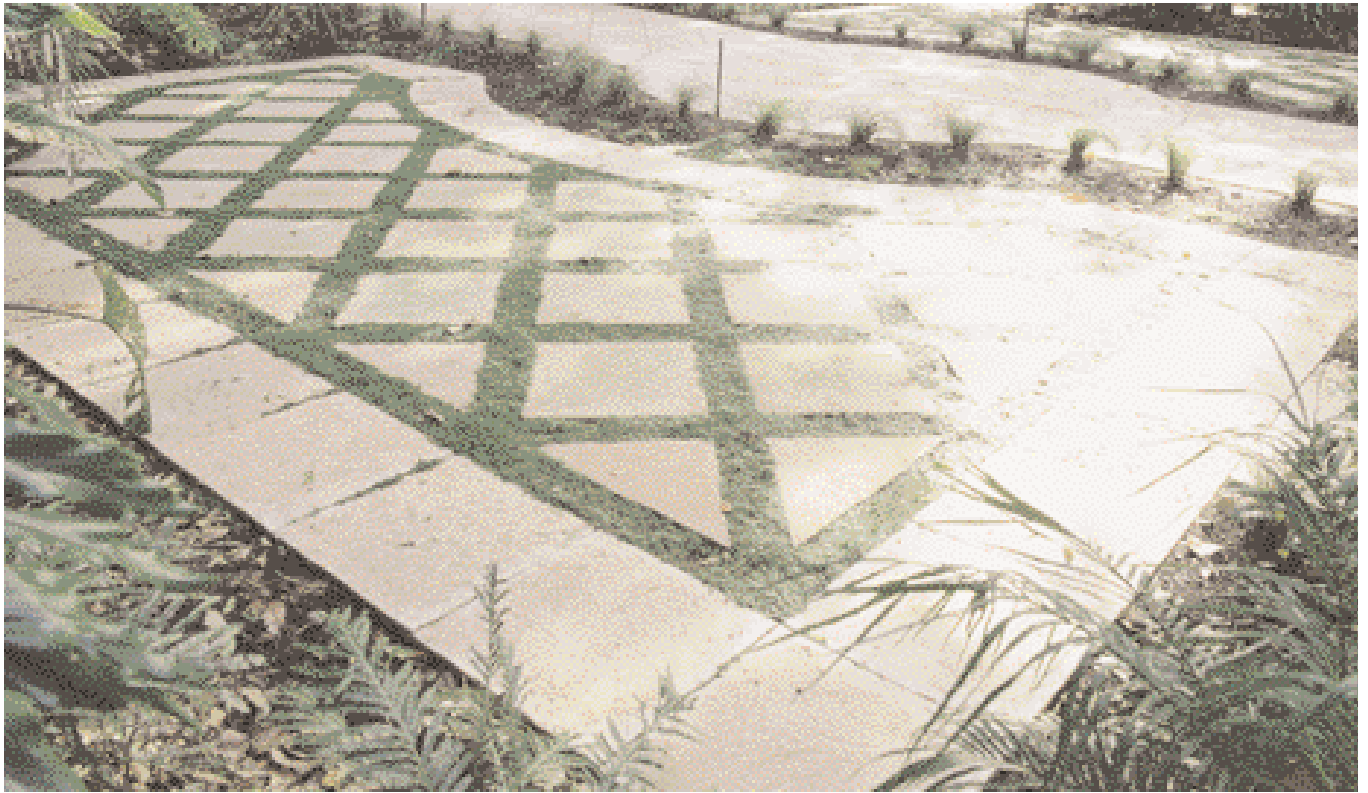
Salmonback Reef paving laid with 100mm gap to accommodate lush mondo grass.
